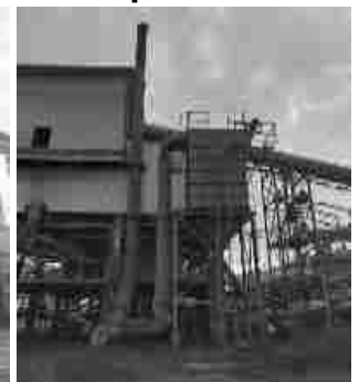
Coal Crusher Bag filter
