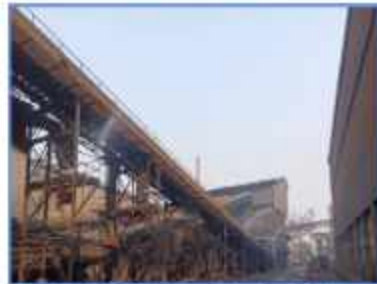
Fixed Water Sprinkler
